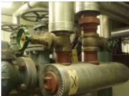
Uninsulated heating valves
