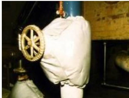
Insulated heating valve
